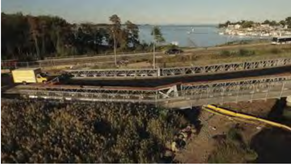
Temporary bridge collapse (October 2015)
